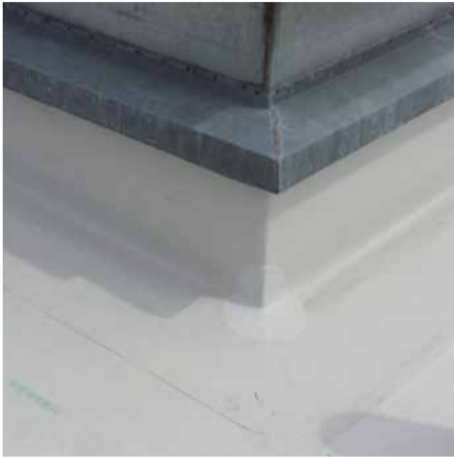
Junctions to right-angled penetrations
